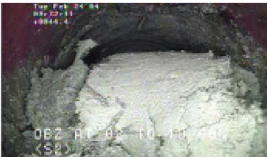
Pictured here: a sewer pipe blocked by grease.
